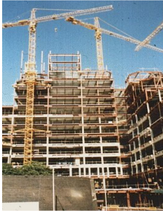
Picture 1 : Typical composite multi-storey steel-framed building during construction - a commercial building in London.
