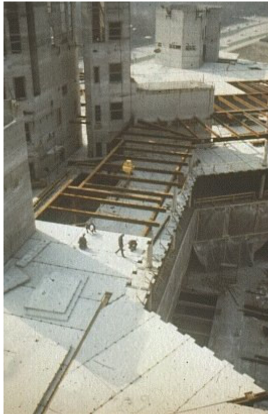
Picture 5 : Instead of an in situ concrete slab, precast concrete floor or deck units can be used.
