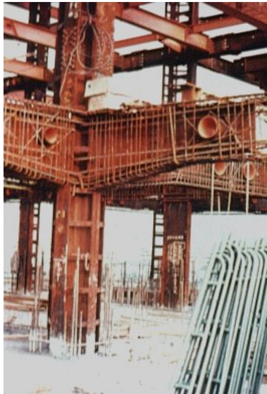
Picture 3 : The combination of concrete cores, steel frame and composite floor construction has become the standard method for multi-storey construction in several countries.
