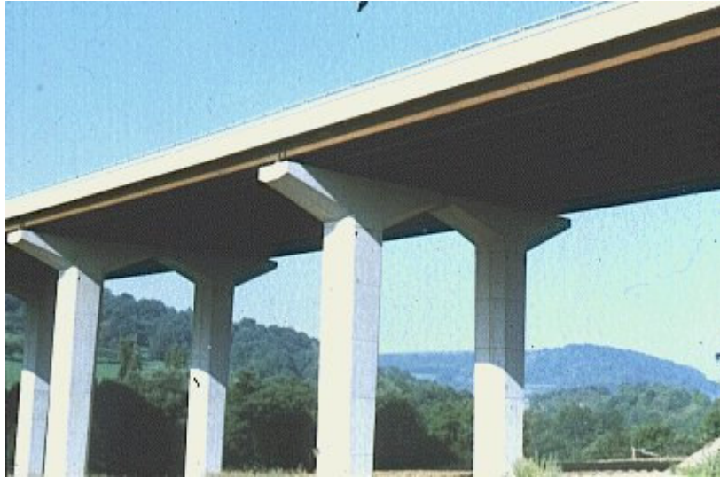
Picture 8 : Medium span composite bridges are normally constructed from welded, built up, steel plate girders and a wide reinforced concrete deck.
