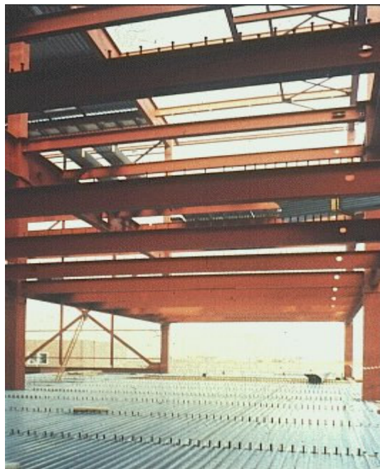
Picture 2 : Typical composite multi-storey steel-framed building during execution - a factory building for the car industry in Germany.
