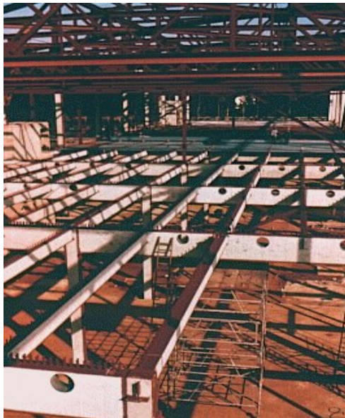
Picture 7 : Partially encased steel sections, for both beams and columns, are an interesting development of the last ten years.
