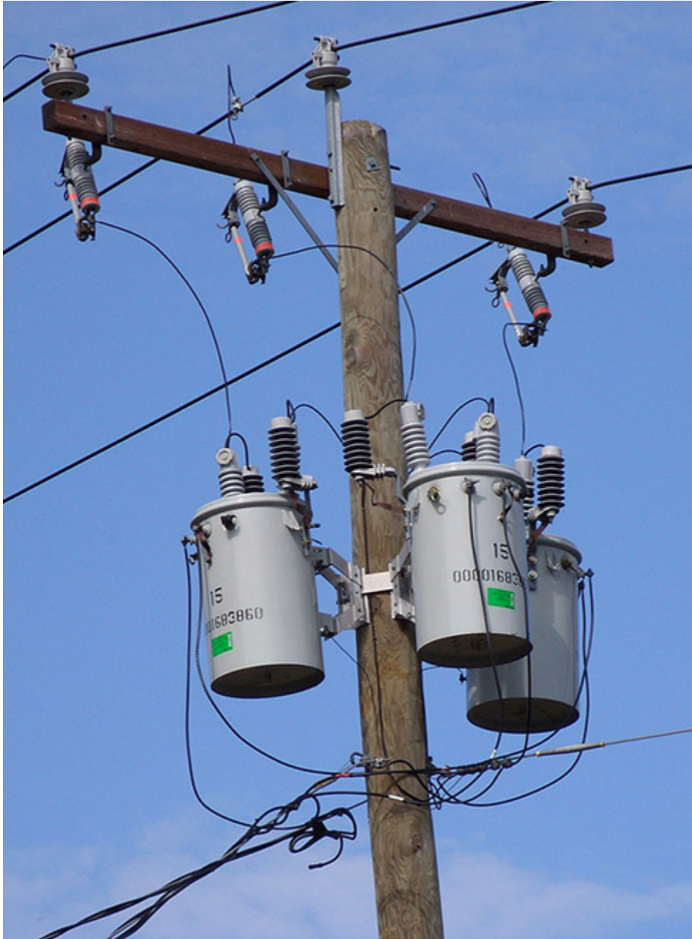
Figure 12.6.2 Transformers are used to step down the high voltages in transmission lines to the 110 to 220 V used in homes. (credit: modification of work by “Fortyseven”/Flickr)
