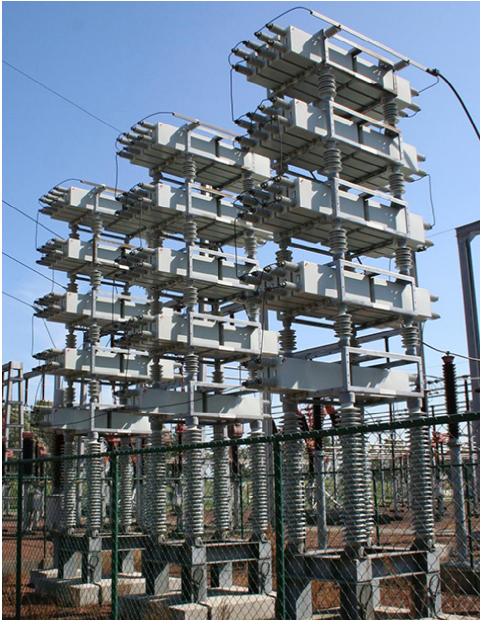
Figure 12.3.4 Power capacitors are used to balance the impedance of the effective inductance in transmission lines.
