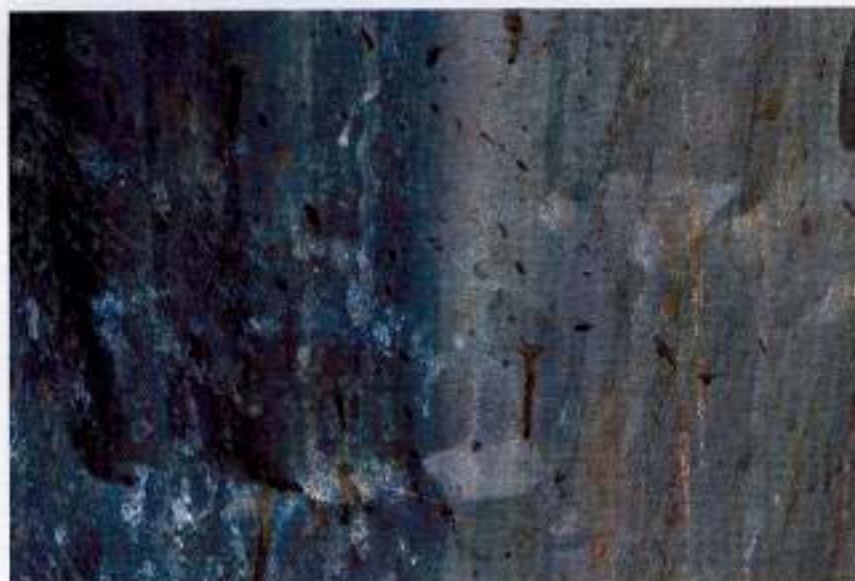
Metal Worn: Galvanized Steel
