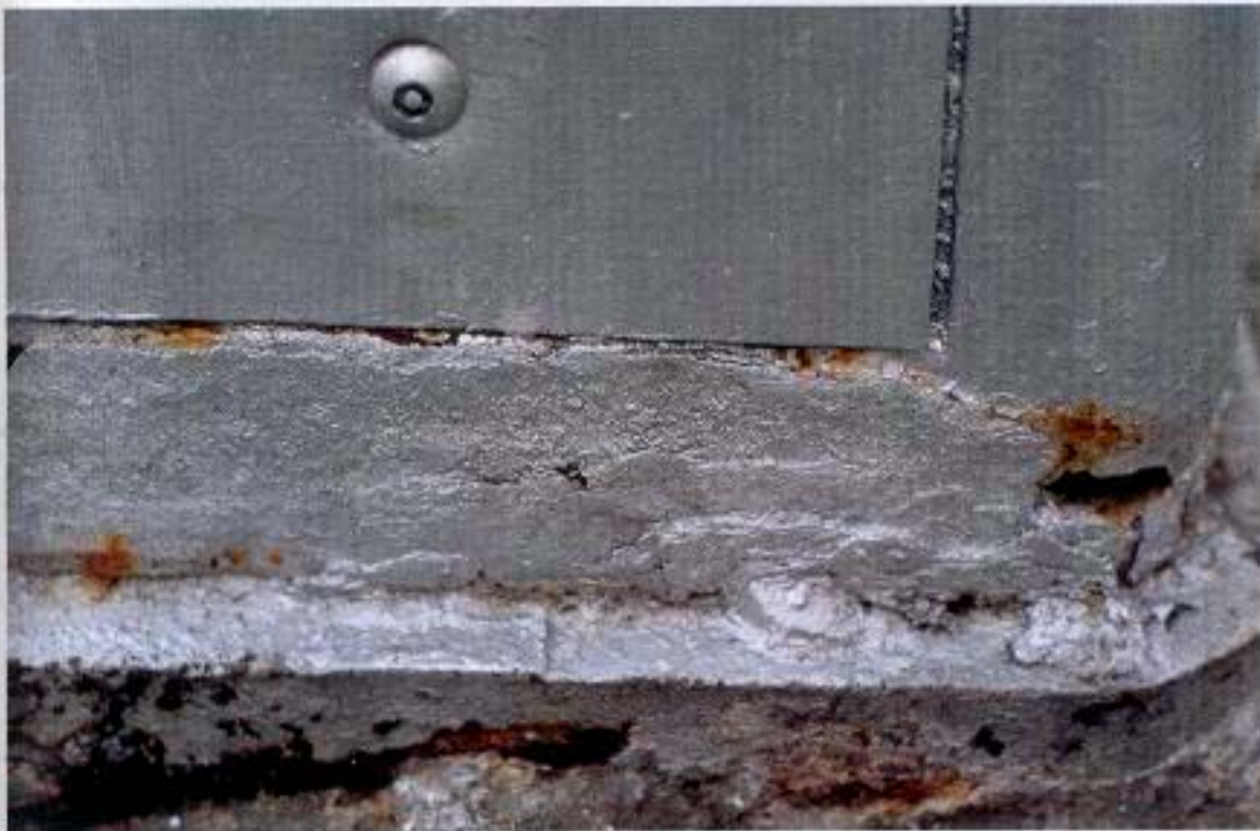
1.10 The rust gives away the material of this lightpost base.
