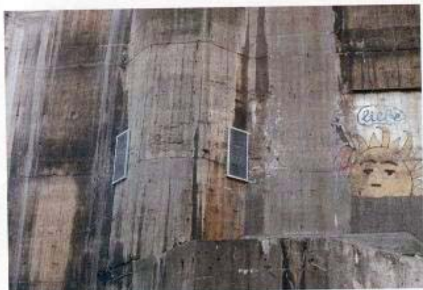
Concrete Worn: Cast Concrete
