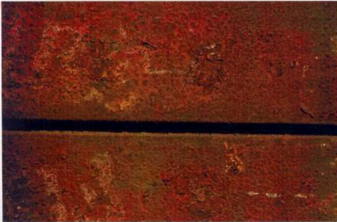
1.4 Rusted metal (Photo courtesy of Brian Drucker).
