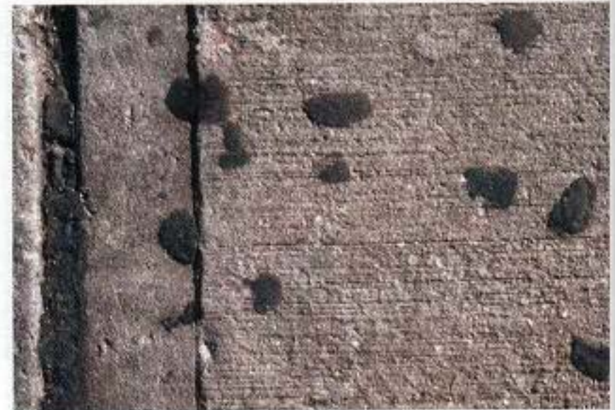
Concrete Worn: Poured Concrete Sidewalk
