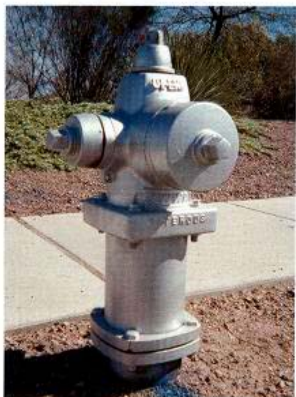
1.5 Fire hydrant in an Arizona suburb.
