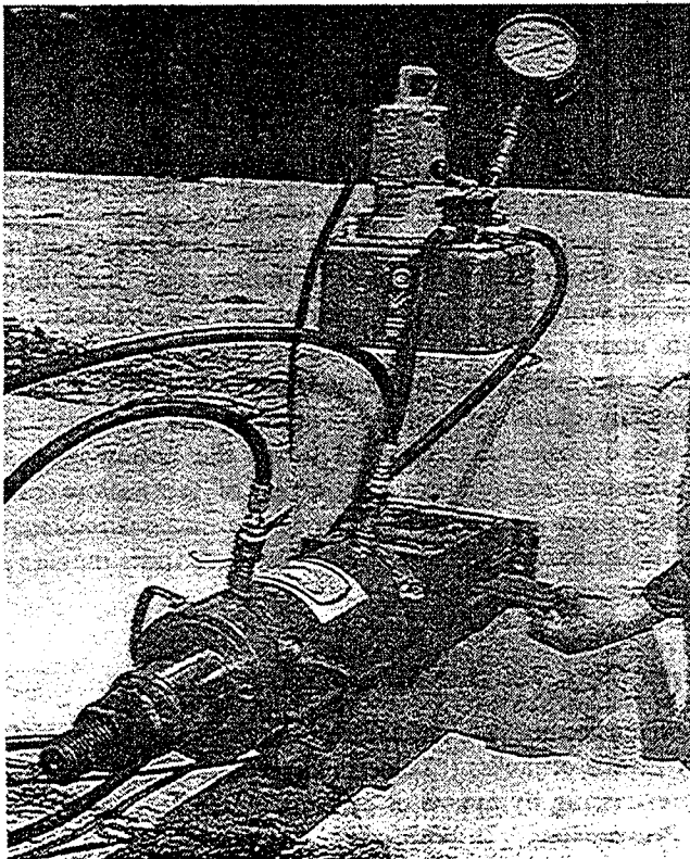
Fig. 3-5. Electric pump operating a hydraulic jack to stress a Prescon cable (note the insertion of shims).
