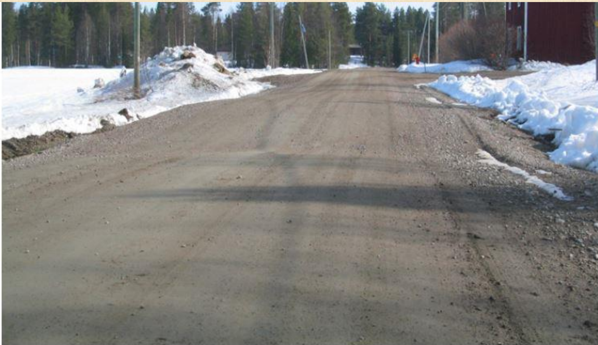
Frost heave problems around culverts can cause unevennesses that drivers feel similarly to bumps.
