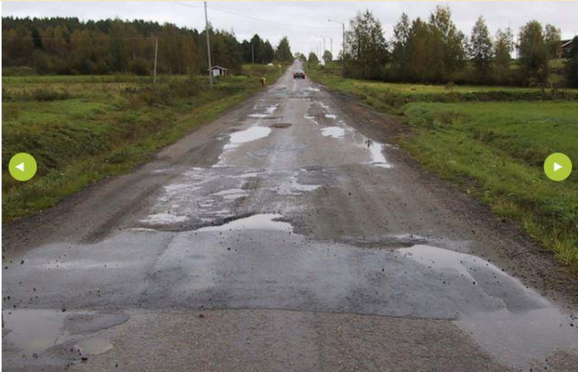
Low volume roads can sometimes be in such bad condition that vibration problems cannot be avoided.
