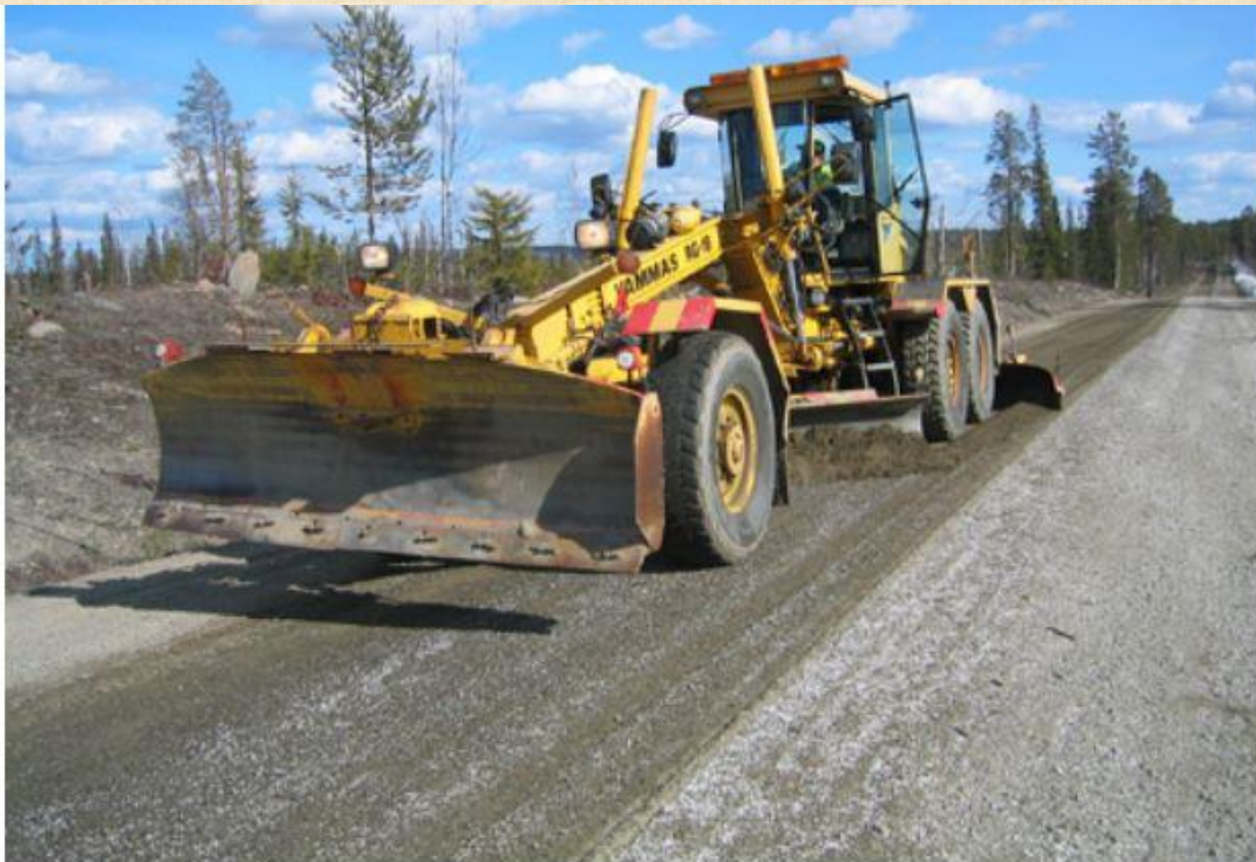
Dust binders can be used in road shaping process to prevent dusting.
