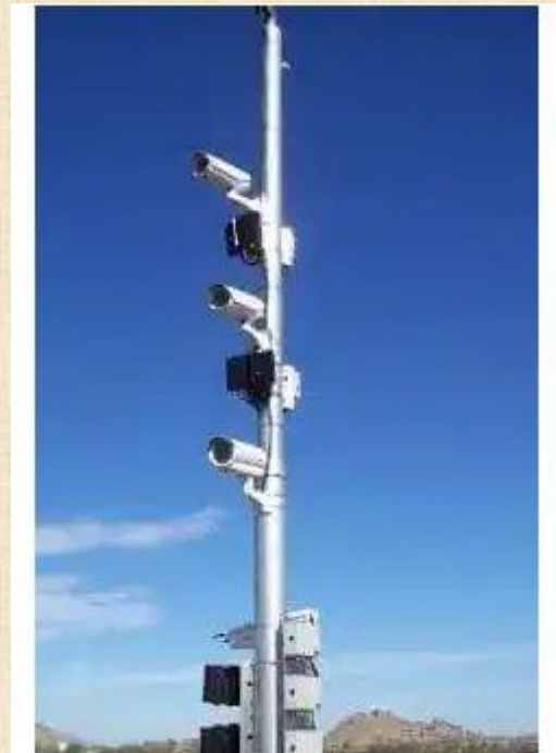
Fig.2: CCTV camera as part of intelligent transportation system
