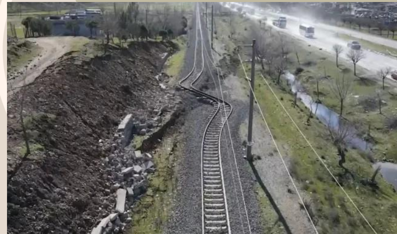
Damaged road and rail tracks
