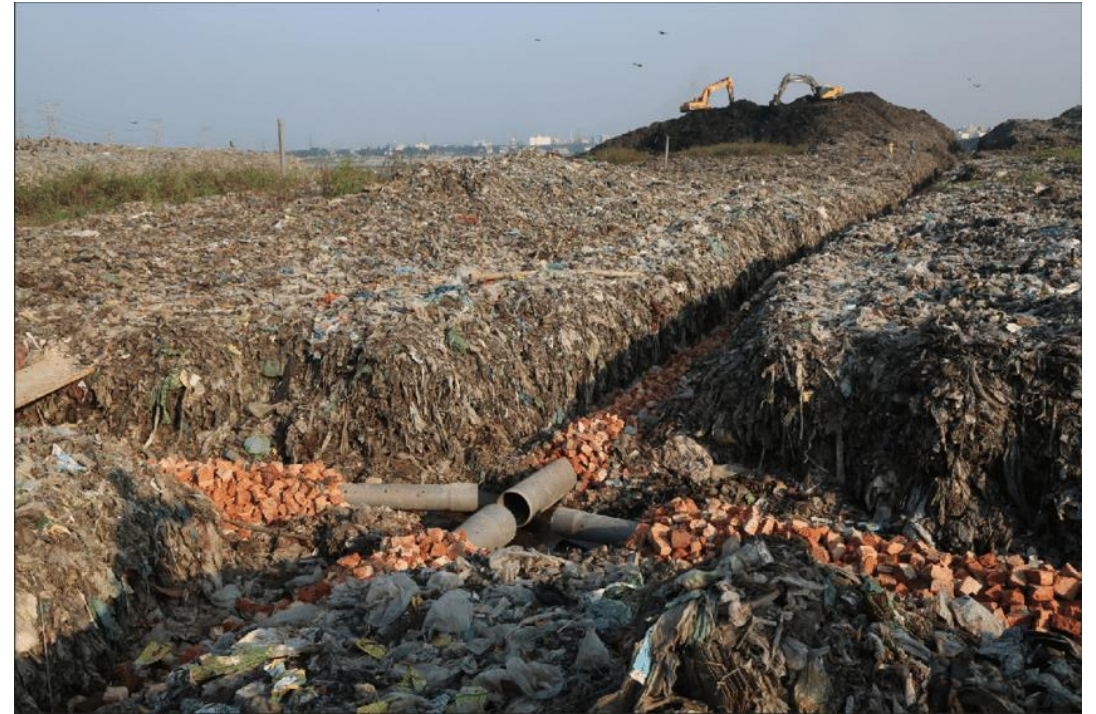
Leachate pipe at Matuail landfill site
