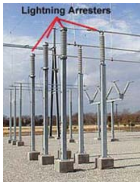
Lightning arresters on bus structures
