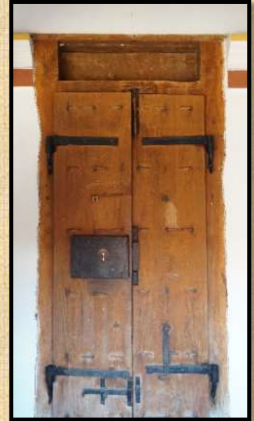
Wooden door with iron battens in tamilNadu. Built with monolithic timber member
